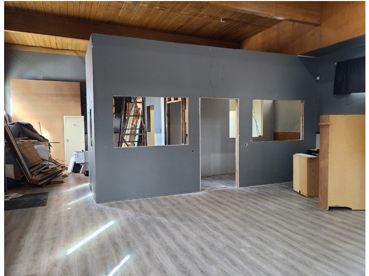
This photo, facing away from the main entrance and open floor space shows an office in front of a washroom and alternate office/storage space.
